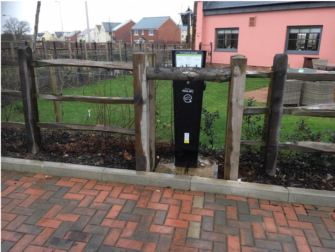
Figure 10 – existing EV charging at Cranberry Farm, Cranbrook
